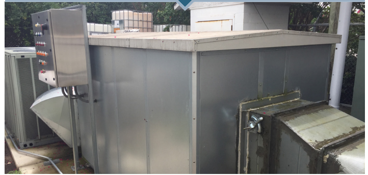
External Feed Ducting
