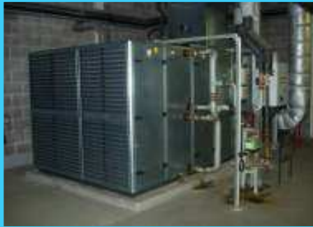
◀ Air handling unit installed at Swansea Bay.
